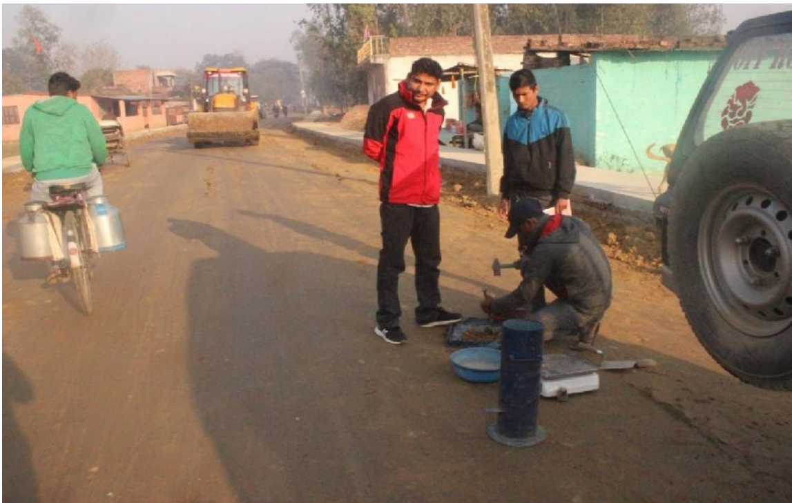
Test of Field Density for Sub Grade at Pilaripur to Rathaiya Nala Road (Balegaon Section), Nepalgunj
