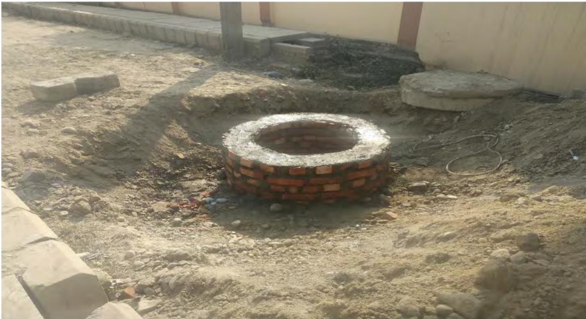
Raising of Sewer Manhole to achieve required design level at R77, Biratnagar
