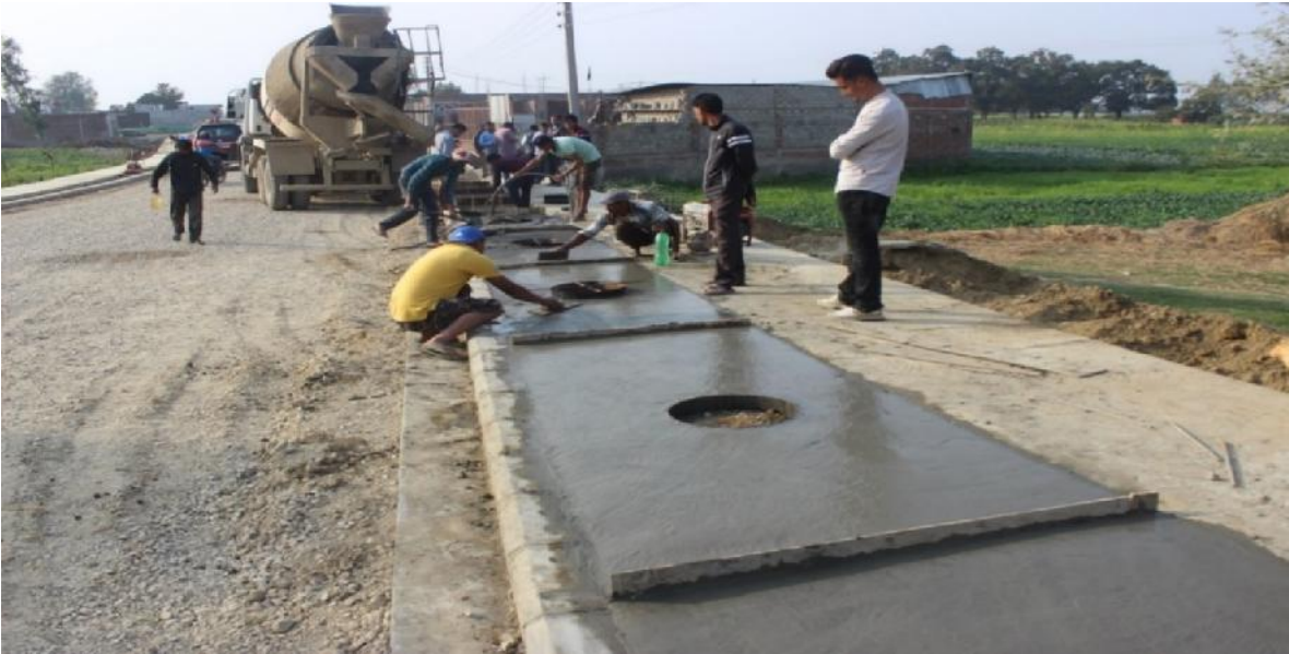
Footpath concrete work in progress at Ganeshman Singh Chowk to Paraspur Road Nepalgunj
